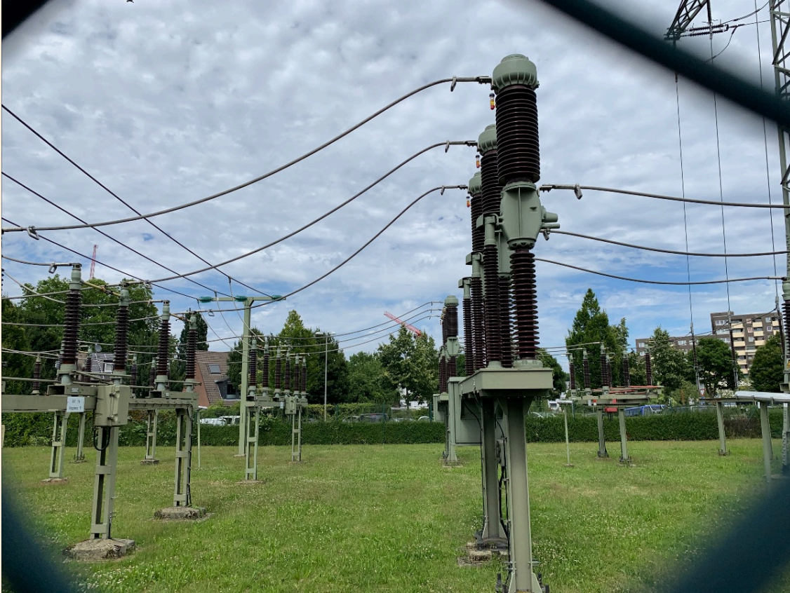
The substation will be central to one of Christina Kubisch's works for The Sound . Photo: Frank Schulte
